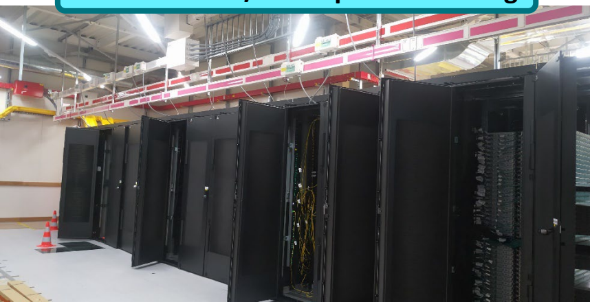
Racks with air/water passive cooling
