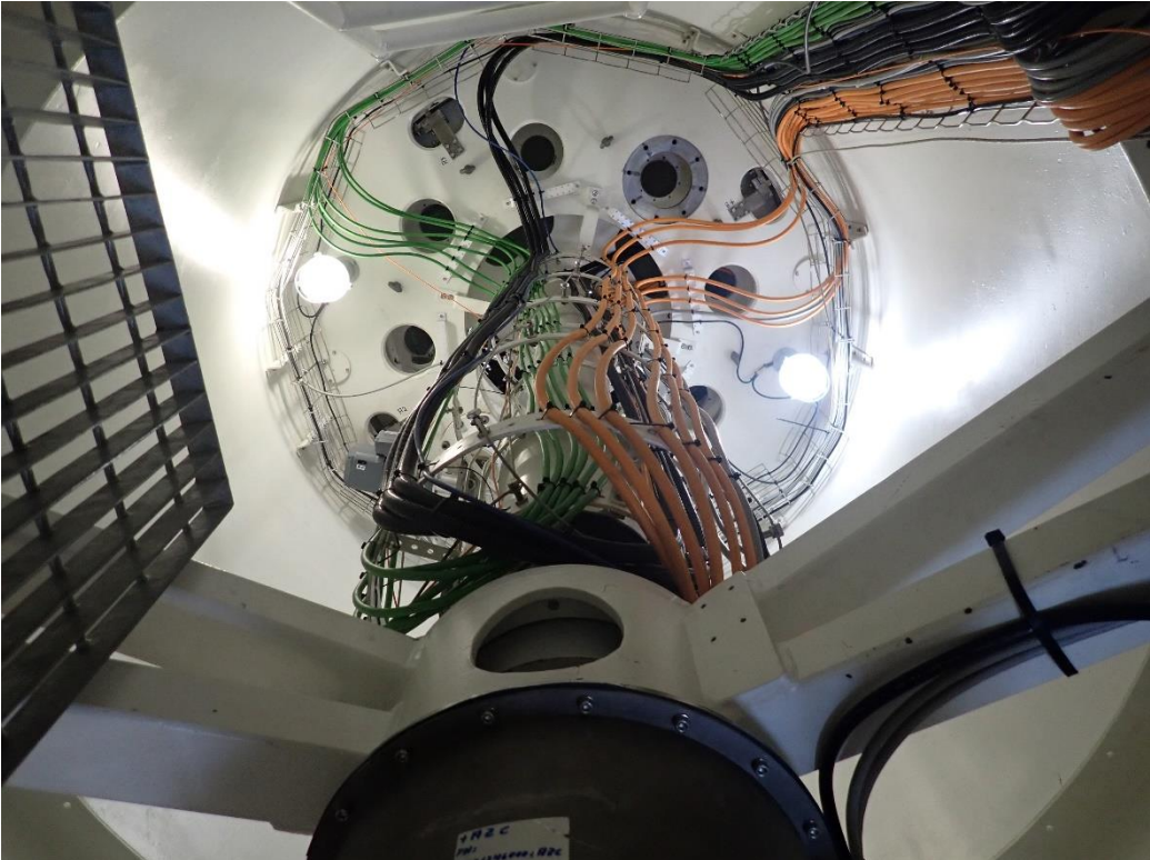
Looking up at Azimuth Cable Handler in the upper part of the pedestal.
